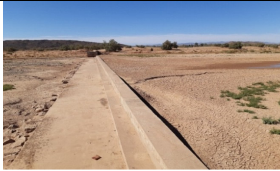
Photo n°3 : Two months after the flood, the upstream of the structure still shows traces of water while downstream, the bed of wadi is dried up.
